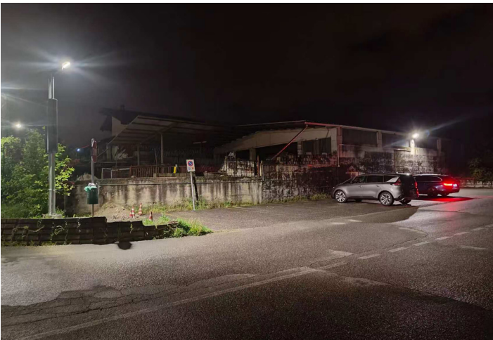
Remote Site & Perimeter Lighting Installed Solar Lighting System: Hera + Galaxia
