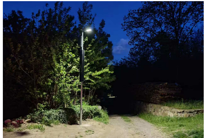
Trail & Recreational Pathway Lighting Installed Solar Lighting System: Hera
