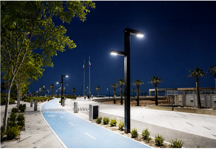
Urban Pedestrian & Pathway Lighting Installed Solar Lighting System: Mars
