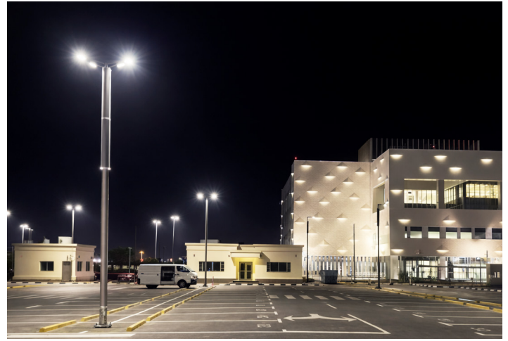
Parking Lot & Area Security Lighting Installed Solar Lighting System: Hera
